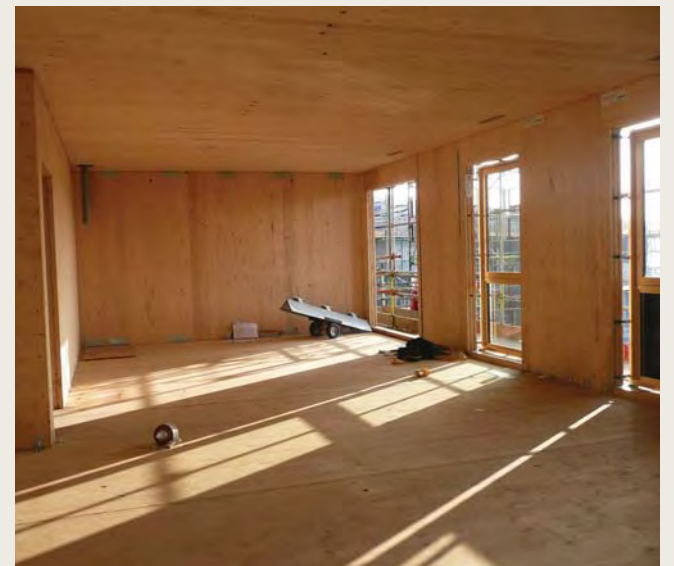
Cross-laminated timber has been used for the floor, walls and ceiling at Bridport House.
